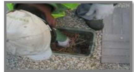
Date: 16.10.2014 Location: Neighbourhood 1 Description: Cleaning valve box
