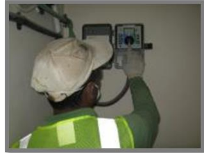
Date: 02.10.2014 Location: Neighbourhood 2 Description: Adjusting controllers
